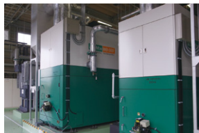
Wood biomass boiler
