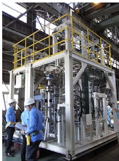
Fig. 3 Photograph of pilot plant for high temperature and high pressure water oxidation (Kimura Chemical Plant Co., Ltd.).
