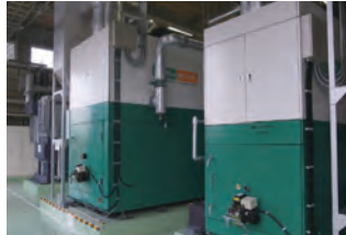
Wood biomass boilers
